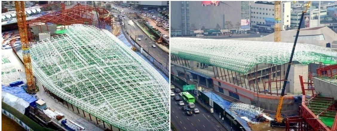
Fig.20. (a) The space frame structure (DLG), (b) The space frame structure (DLG) with concrete columns and walls
