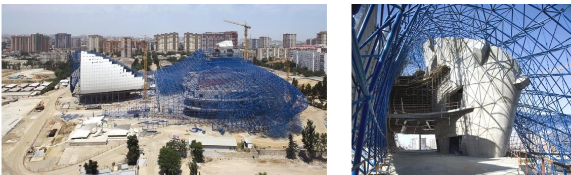
Fig.12. (a) The space frame structure of Heydar Aliyev center, (b) Steel and RC materials used in structural system of the center
