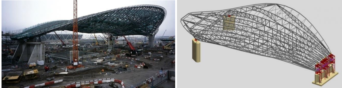
Fig.3. (a) RC wall with RC columns supporting the space frame structure (DLG), (b) Illustration of DLG with RC wall and RC columns
